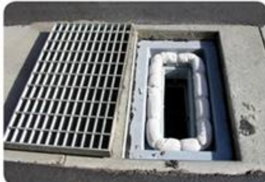
The grate inlet skimmer box is an expensive and high maintenance method of filtering stormwater. These holes are generally categorised as high-tech green solutions.
