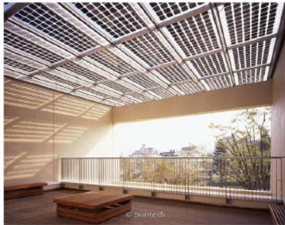
Fig. 4. Glass ceiling with transparent BIPV modules [21].
